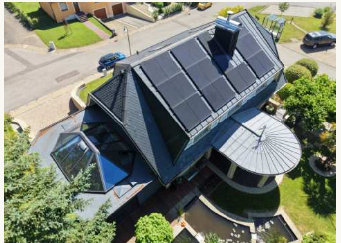
Rooftop solar panels
